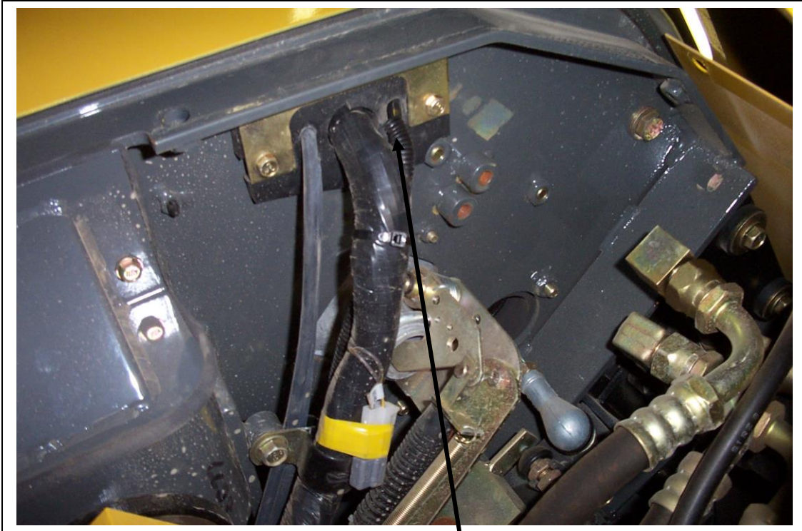
Two wires to A/C on off switch going up through the floor at the front right corner of the cab.
